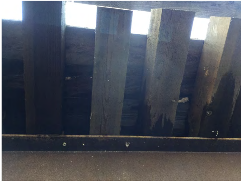
Indications of rot in subdeck, surface rot only
