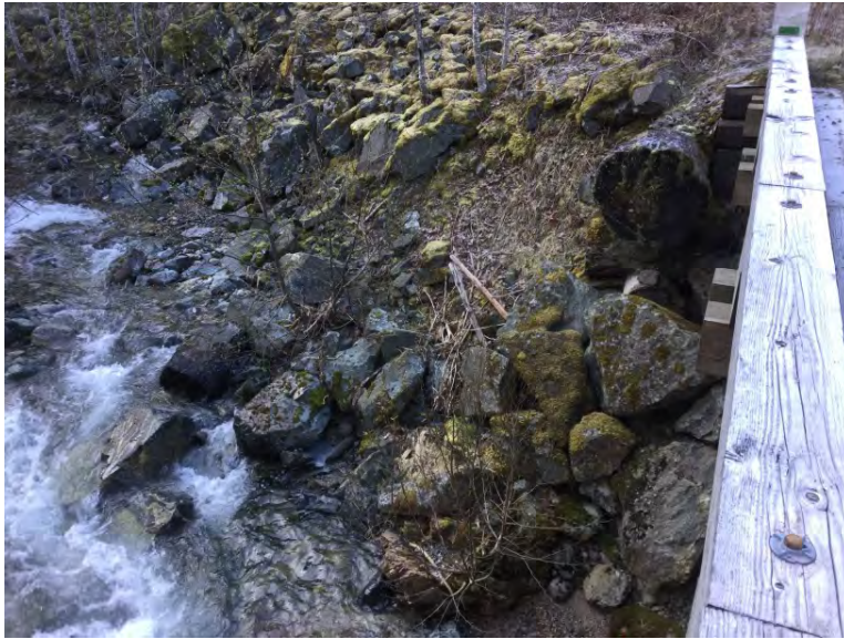
Upstream left bank riprap scour
