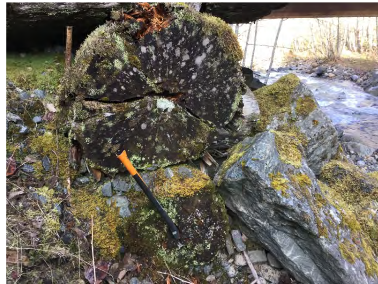
Upstream face log ends are rotten
