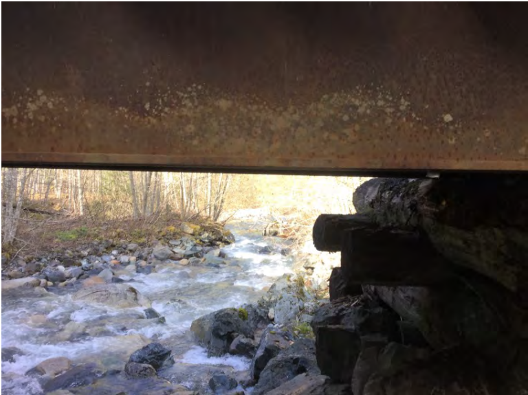
Approx 10mm settlement of downstream girder at right bank
