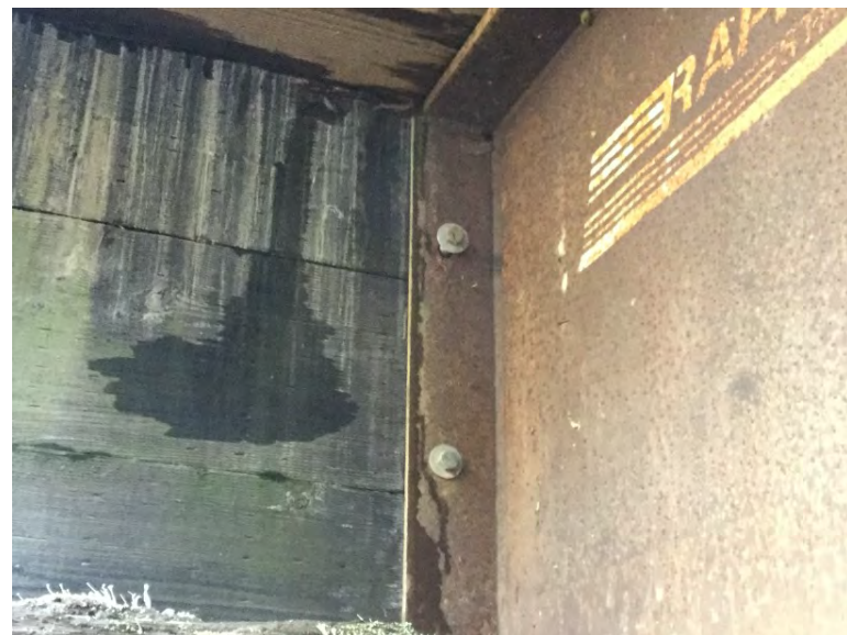
Ballast wall to girder connection loose
